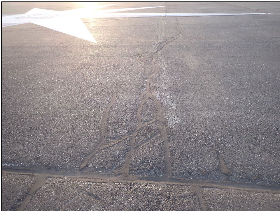
AP-04-04: Alligator Cracking
