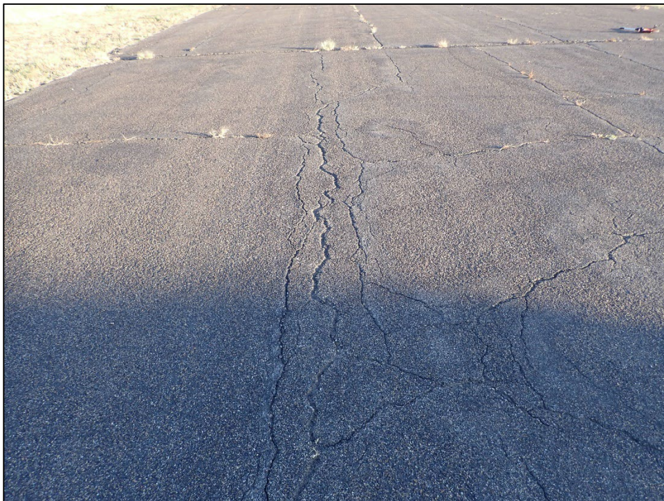
TW-01B-10: Alligator Cracking
