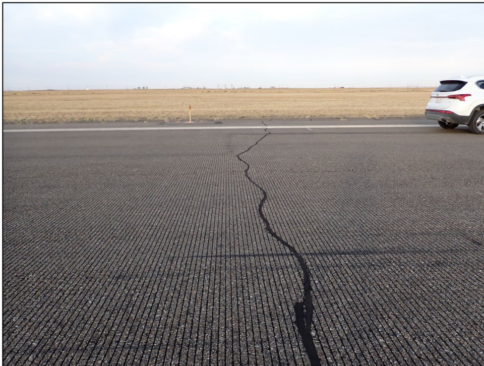
RW13-12-76: L&T Cracking
