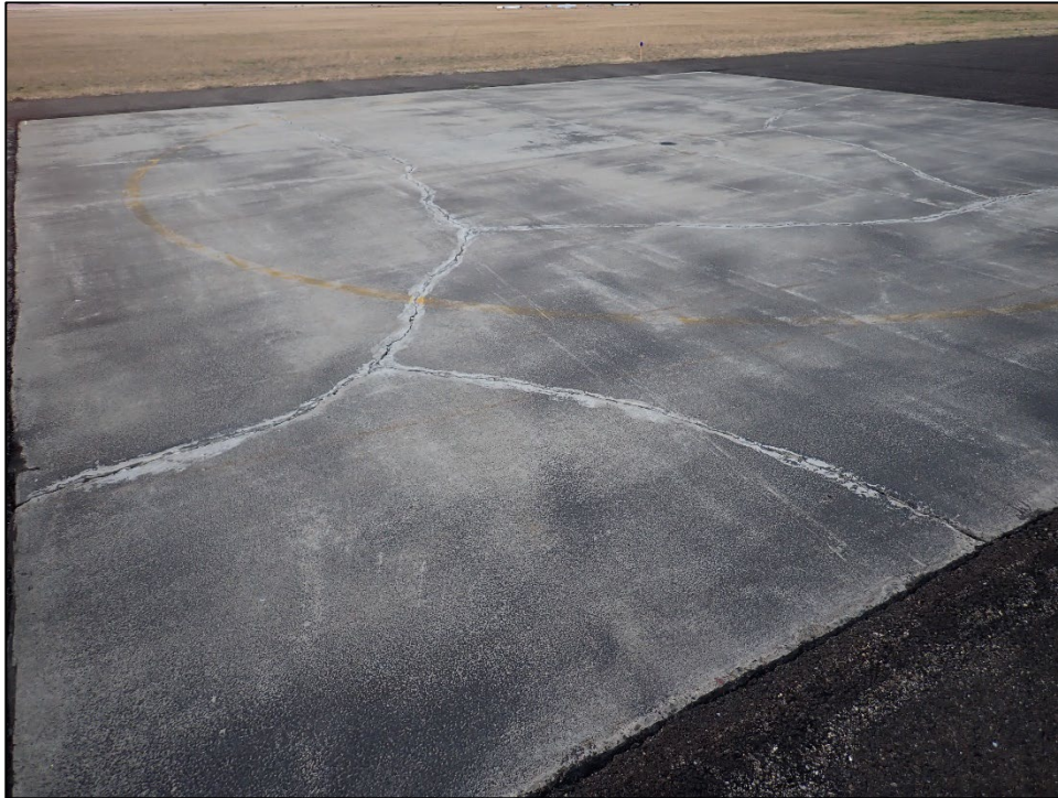
AP-05-01: Shattered Slab/Intersecting Cracks
